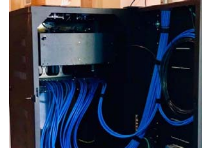
Telecom & Wireless Access Point Technology Upgrades Completion Fall 2019
